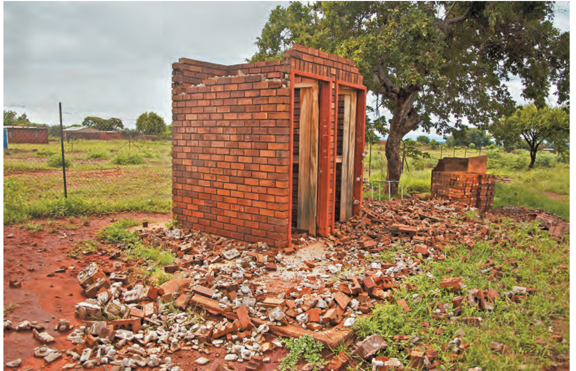
The dilapidated pit latrine brick structure had been built by parents in the 1990s and shared by both boys and girls. Boys also used an open-air urinal close to the toilet to relieve themselves.
