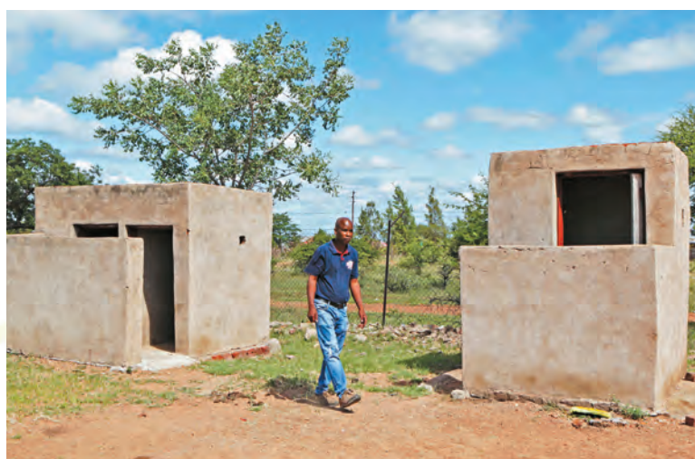
Long queues formed outside the old pit latrines, forcing some pupils to opt for the bush behind the school to relieve themselves.
