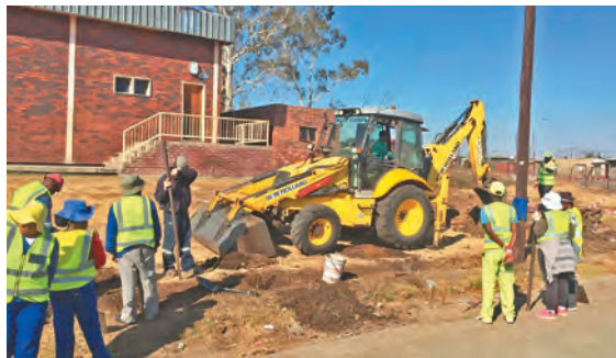
Contractors are hard at work building a security house and safe parking ports.
