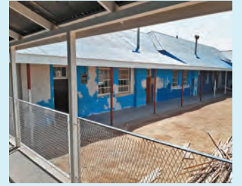
Paint on the walls was peeling off, making the premises look unappealing.
